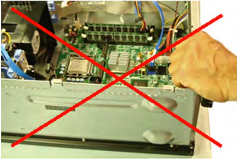
Figure 10. Chassis "Bare Metal" Grounding (Unacceptable)
