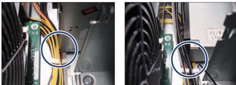
Figure 59: Routing power cables with installed LTO drive
